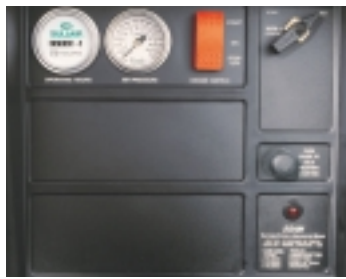
Curbside Instrument Panel With (SSAM) Shutdown System & Annunciation Module.
